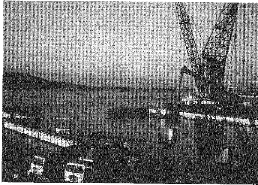
Fig. 3--View of the jobsite during underwater placement -- concrete is pumped from the truck mixer to the tremie hopper from which it flows to the bottom of the sea through the pipe
