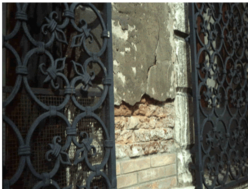
Fig. 4 – Detachment of a cementitious rendering mortar due to ettringite formation according to equation [1] for the presence of \text{SO}_4^{=} in the bricks of the masonry wall.
