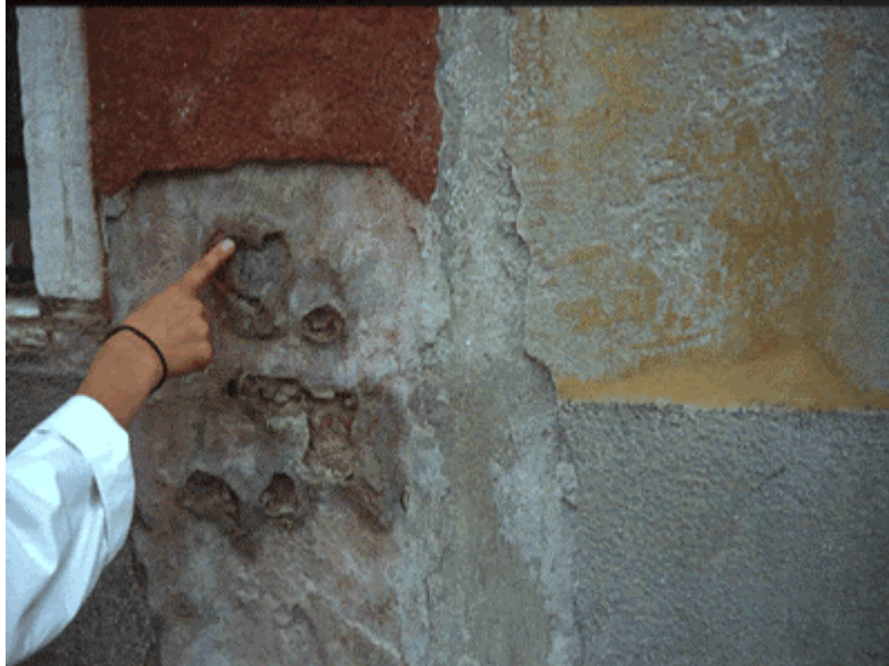
Fig. 5 – Severe damage of the rendering mortar (on the left) due to NaCl crystallization and thaumasite formation according to equation [2], both caused by capillary rise of sea water in Venice. No damage in the wall on the right for the barrier against capillary rise.
