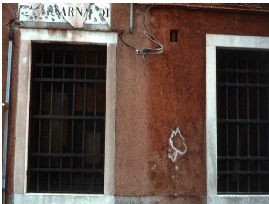
Fig. 2 – Typical efflorescence defect caused by NaCl crystallization on the masonry wall in Venice.
