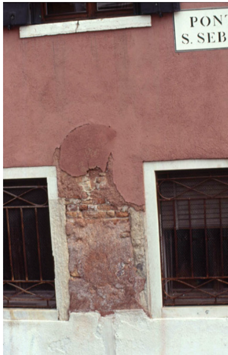
Fig. 3 – Typical subflorescence damage due to the detachment of the rendering mortar.
