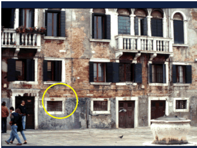
Fig. 6 – Cementitious mortar on the wall of a building in Venice to protect it from the sea water during the high tide.
