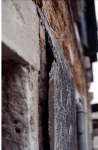
Fig. 7 – The mortar shown in Fig. 6 completely detached from the wall due to restrained expansion related to swelling and NaCl crystallization.
