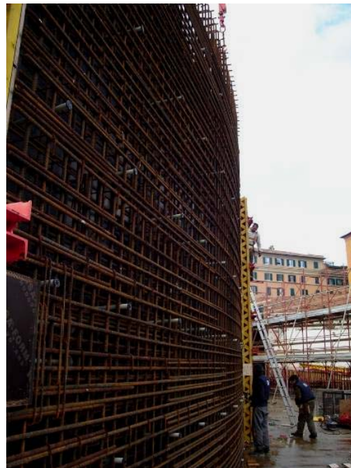
Figure 8 – Example of steel congestion in a typical wall of MAXXI, Rome, Italy
