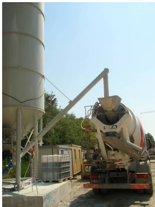
Figure 14 – Supply of the expansive agent at the jobsite with an automatic silo
