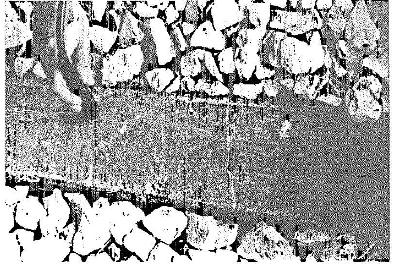
Fig. 5 - Use of optical microscope for field experience to detect microcracking in concrete ties in service.
