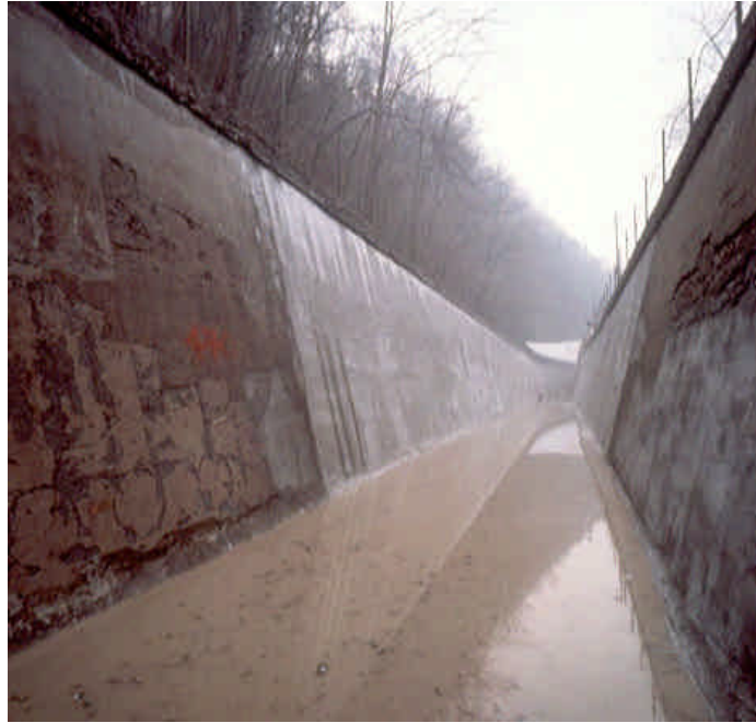
Figure 23 - Cracks promoted by excessive strain-induced tensile stress from shrinkage in the surface of the cementitious material.
