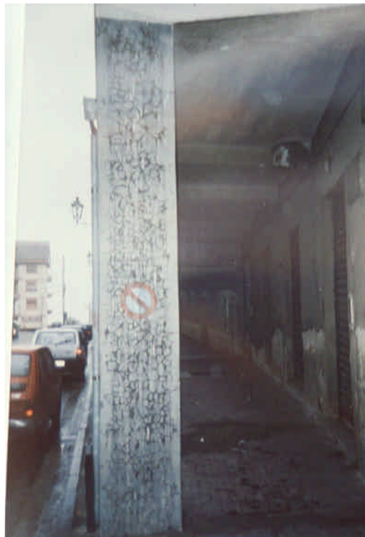
Figure 24 - Cracked enlargement manufactured with high-strength shrinkage-compensating mortar.
