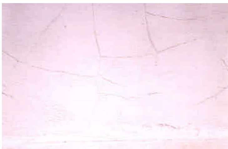
Figure 22 - Cracks on the surface of the shrinkage-compensating mortar used in repairing cooling tower in Fig. 21.
