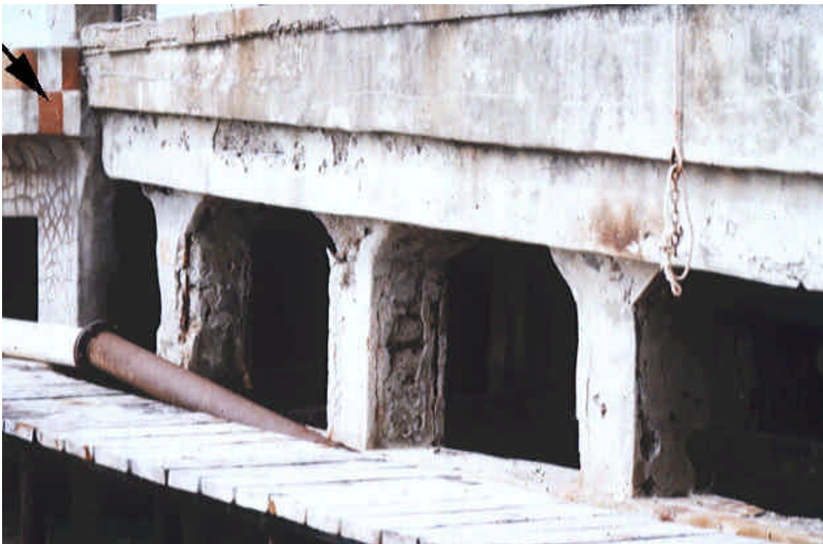
Figure 20 - Crack patterns in a marine structure repaired (on the left) by using high strength shrinkage-compensating mortar.
