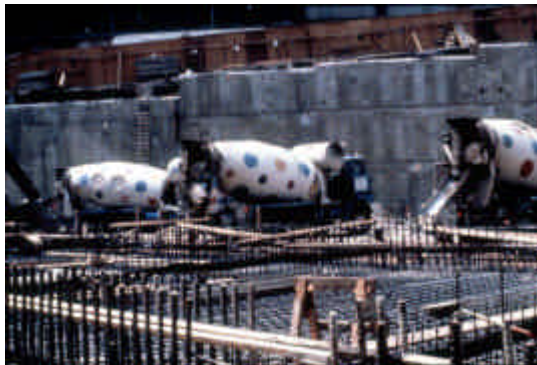
Fig. 8 - Placement of self-compacting concrete in a reinforced slab foundation of a skyscraper (Commercial Center) in New York (1978).
