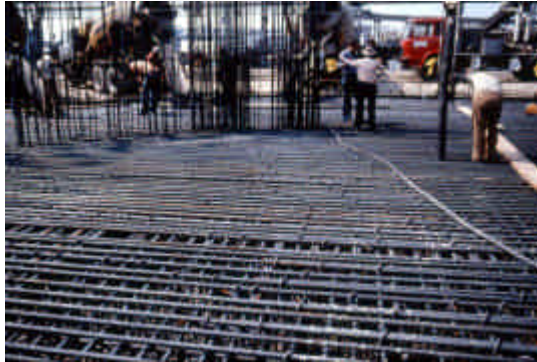
Fig. 7 - Congestion of reinforcements of a slab foundation where concrete (on the background) is placed without vibration [8].
