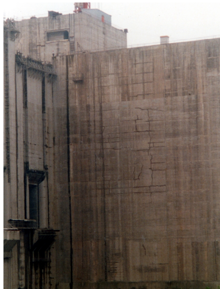
Fig. 6 – Thermal-related cracking in the first placement with concrete combining the SN-based superplasticizer [10].
