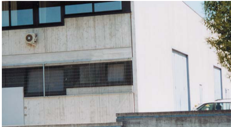
ig. 13.5 – Dark surface on the left site of the building and white surface on the right
